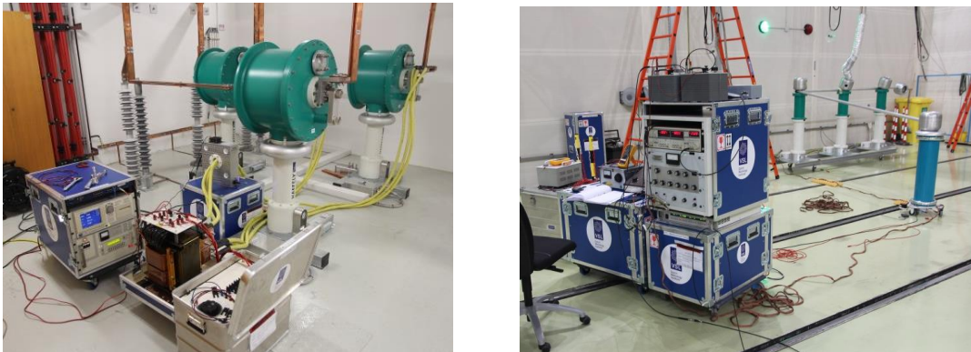
Figure 4: Pictures of an actual on-site LMS component calibration of the current channels (left) and voltage channels (right), using a sampling current ratio bridge and a high-voltage capacitance bridge respectively.
